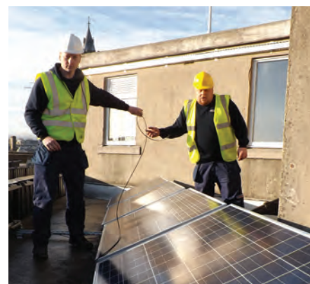
Rooftop solar panels
